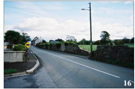
Photo 16: Stone wall on the Callan Road requiring repair.
