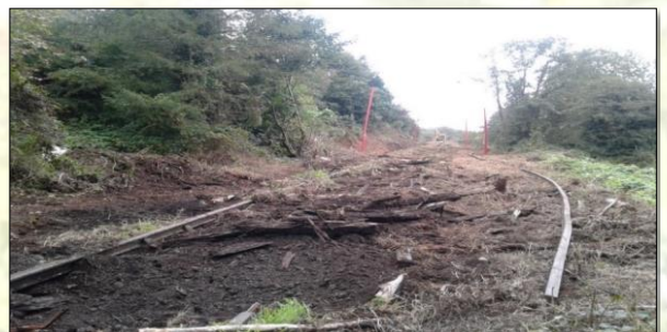
October 2020 - Lifting of old rails and sleepers along the route of the South East Greenway
